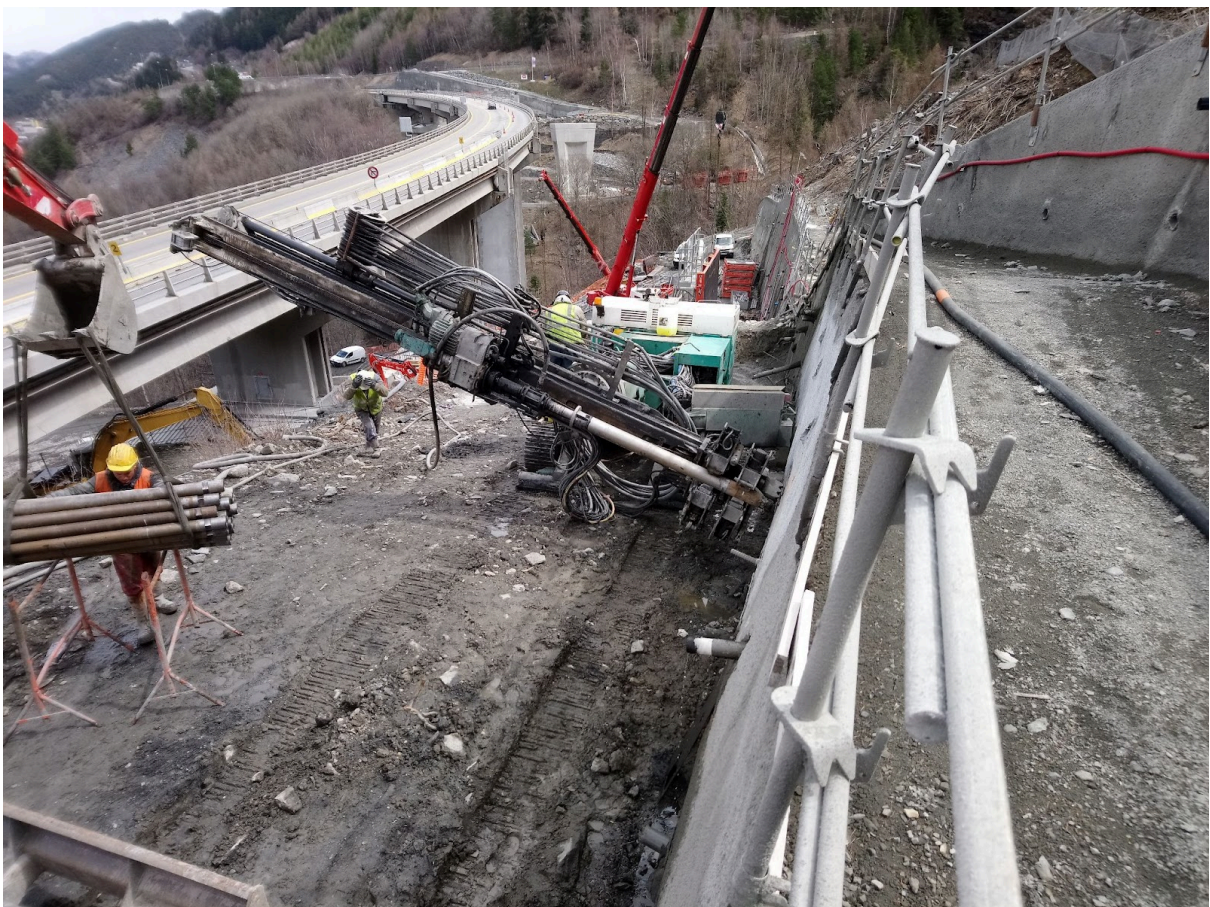
Excavation of access cuttings to the new Charmaix viaduct, drilling of nails
