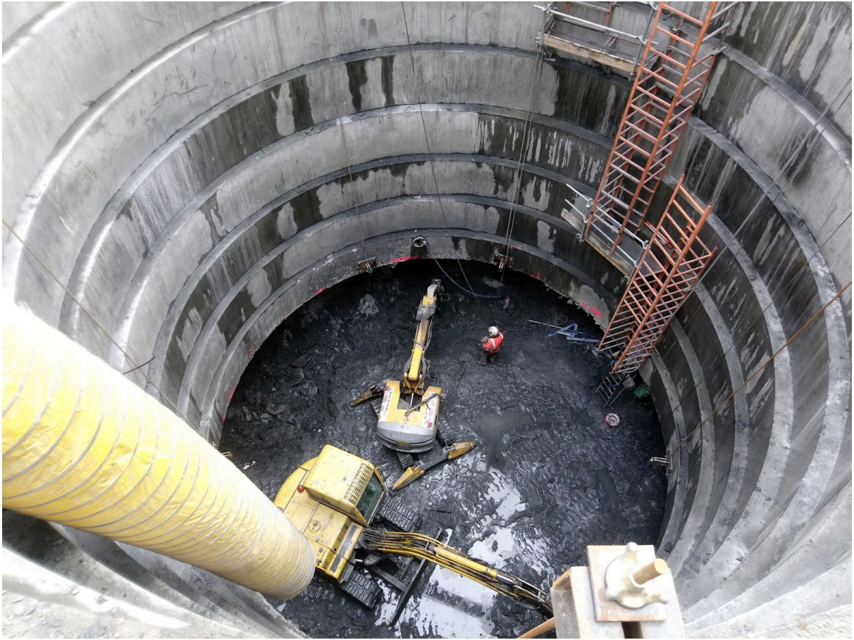
Realization of the Moroccan well for the future fixed P2 pile of the new viaduct
