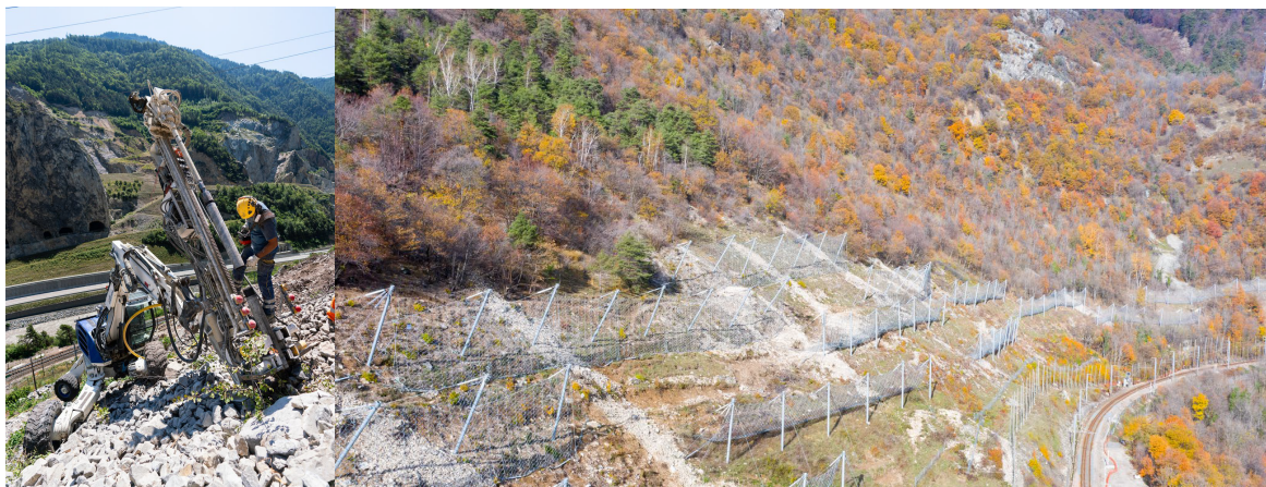
Protective devices - La Saulcette slope
